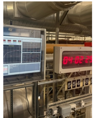
Recording of Fire Test Exceeding 4 Hours Duration
