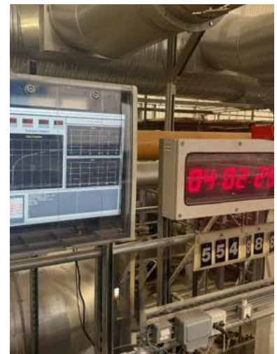
Recording of Fire Test Exceeding 4 Hours Duration
