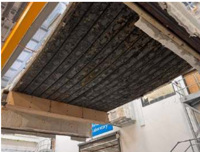
The exposed face of the floor assembly immediately after the test
